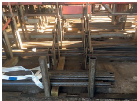
Pockets with uneven fall lines, limited fall reduction and boxed steel posts
